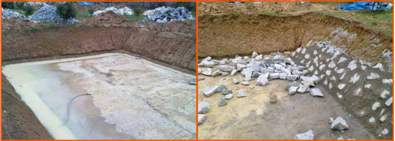
Figure 12: Construction progress, laying the concrete floor and linking the walls with riprap for BR1
