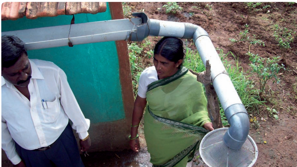
MYKAPS: Harvested rainwater for sanitation needs
