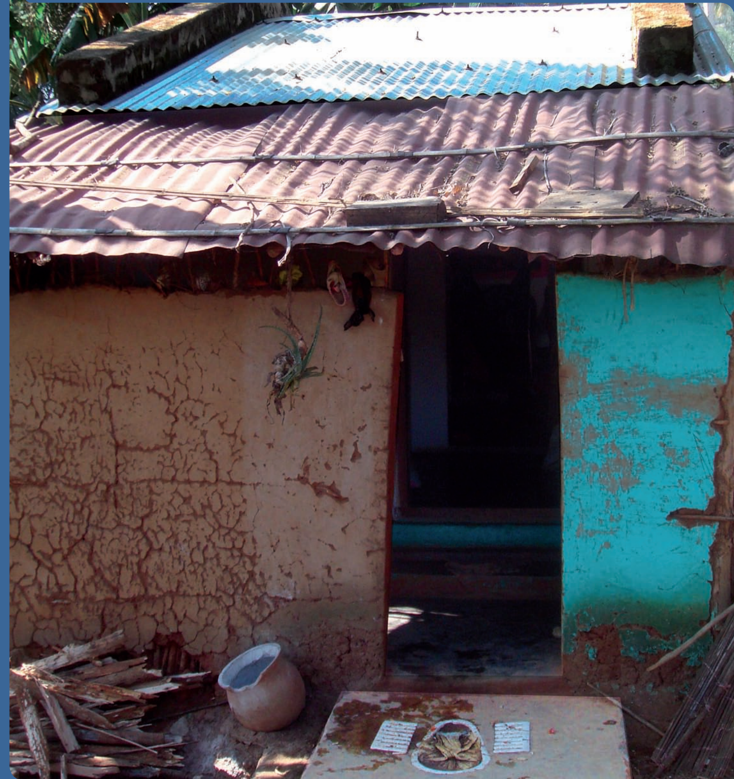
IMAGE 3: All sides open, at the doorstep: An unusable toilet in Orissa
